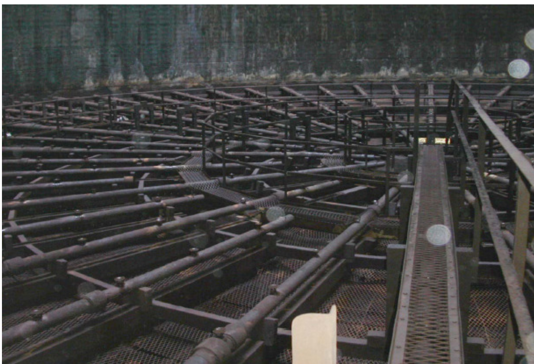
Figure 3.17: View of the X-Grid layers inside the cooling tower after 20 years service. Diameter is approximately 52 meters (NN 2007).
