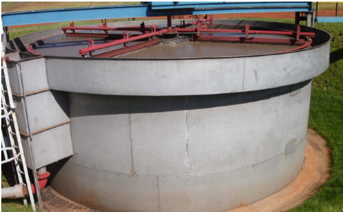
Figure 3.12: DAF Thickener built in 1989 for the Middelburg Municipality (NN 2007).
